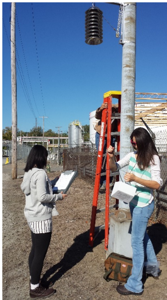
Figure 55. Installation of benzene passive samplers
